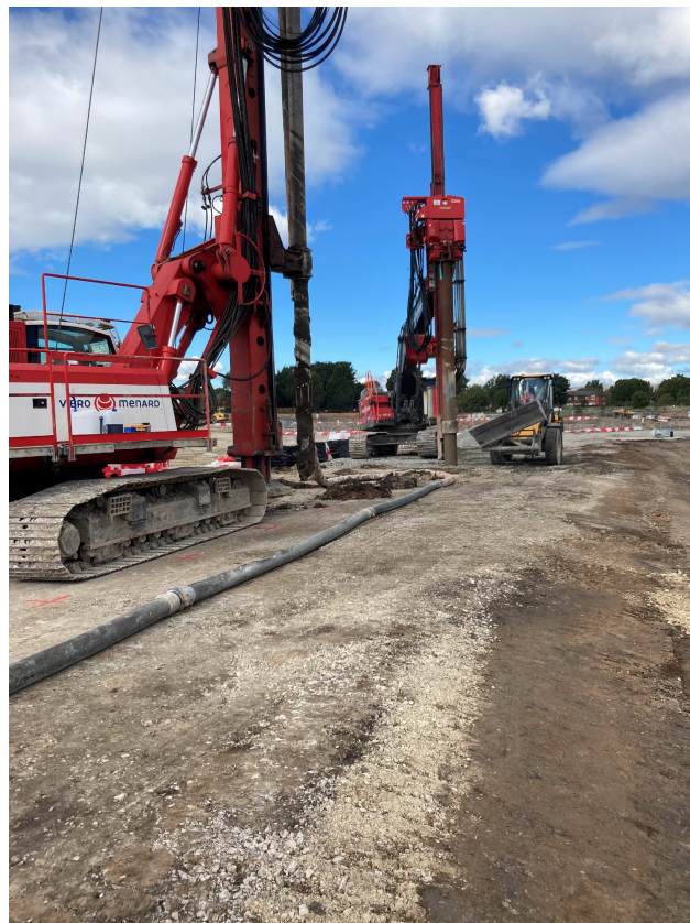
Figure 5 - BMC Setup on site
